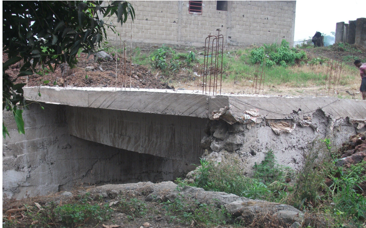
Construction of the community bridge in Buea, selected as a priority project in agreement with the Council and Communities
